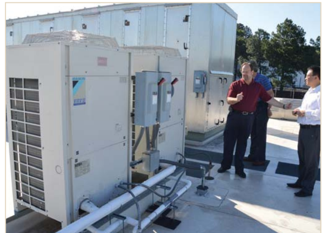
One of the 14-ton VRF heat recovery units mounted on the roof of the ASHRAE headquarters building.
