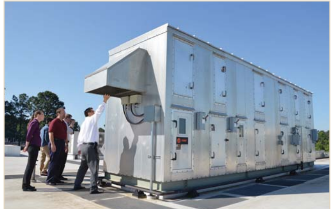
The dedicated outdoor air system.
